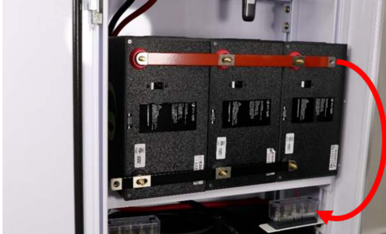
Figure 8.0 - PHI Battery Wiring Using Interconnecting Busbars
