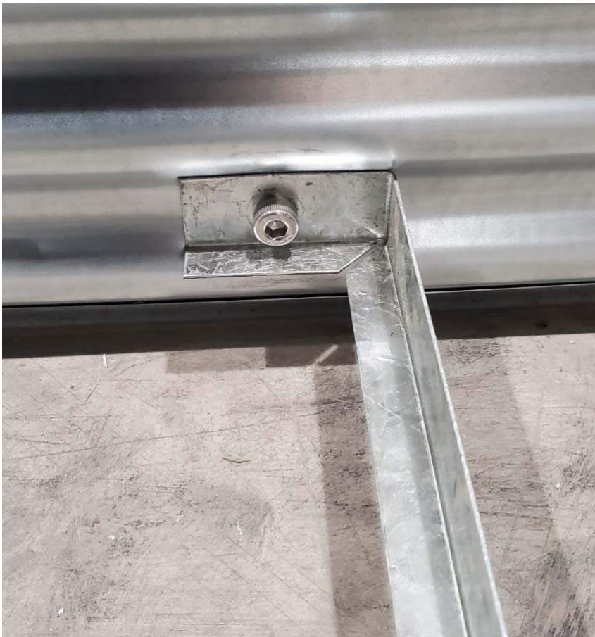
Fig 5. – Cross Brace installed on the inside face of the Long Side Panel
