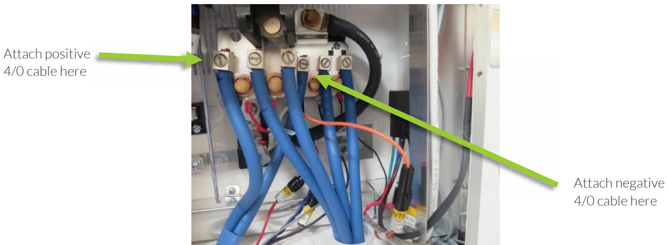
Figure 10 – 4/0 Cables Landed in the Conext Mini PDP (AccESS – Schneider)
